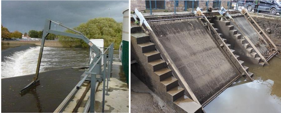
Figure 5.3 Screen cleaning in the DDC. (Photographs: Author, 2020-2023) Derby, new HEP installation rake system (2012) Belper, Rake and chain self-cleaning screens (2015)
