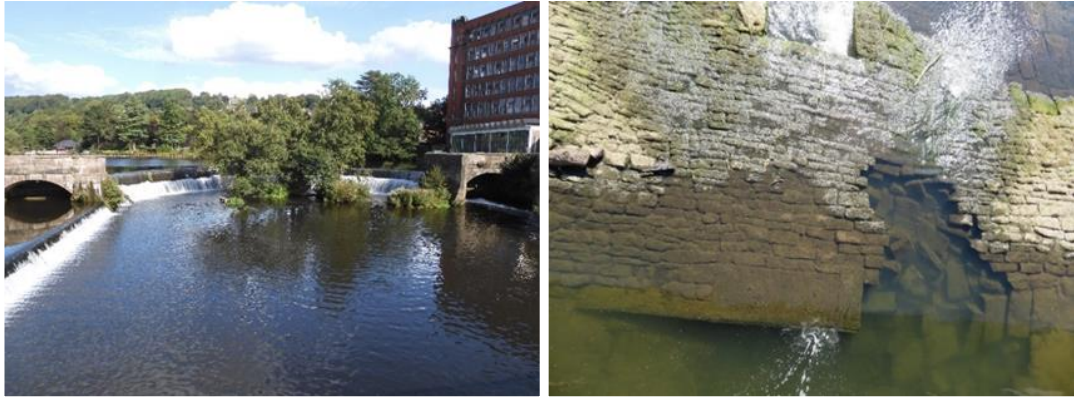
Figure 5.22 Belper circular and northside weirs.. The secondary 'Rock weir', right, with a hole (possible tunnel collapse) (Photographs: Author, 2023 2018)
