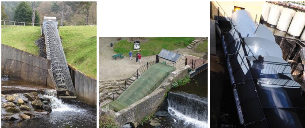
Figure 5.2 Archimedes screws generating HEP at Cragside (Northumberland), New Mills (Derbyshire) and Borrowwash (Derbyshire) (Photographs: Author 2020-2023)
