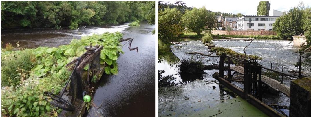
Figure 5.23 Sluices in a state of disrepair on the River Derwent, Baslow (left) and Milford (right) (Photographs: Author, 2023 2020)
